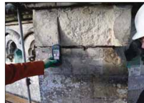
Corroding cramps causing damage to buttress masonry
