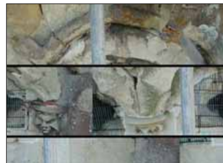
Setting out resulting in mis-alignment
